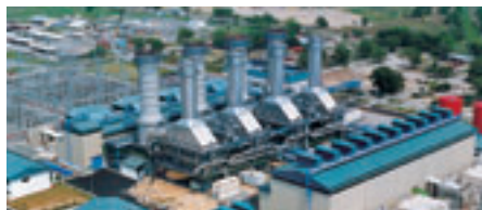
Paka, Malaysia: 404 MW combined cycle power plant consisting of two blocks with two V94.2 (new: SGT5-2000E) gas turbines each
