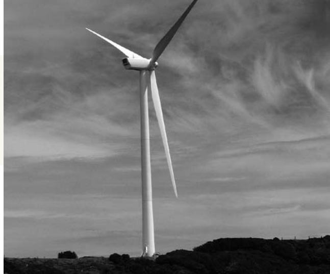
Tararua Windfarm, Manawatu
