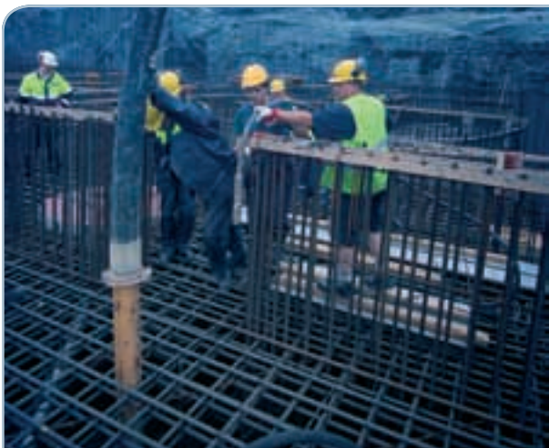
The top photo shows the reinforcement steels of the reactor building and the bottom photo the concreting of the base slab for the fuel building.
