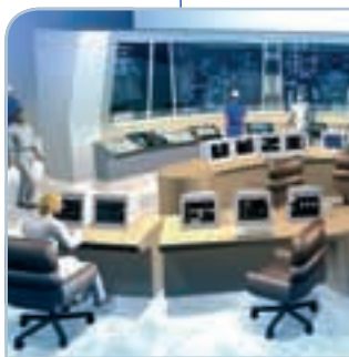
The OL3 control room is of ergonomic design with four separate working areas for reactor and turbine operators, shift supervisor and systems and screens to show a plant overview.
