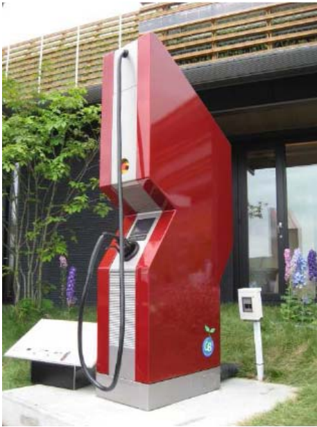
Figuur 6-2 Fast charging station van Tokyo Electric Power Company (Bron: http://www.iea.org )
